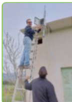
Wireless networks (e.g. LoRaWAN)
